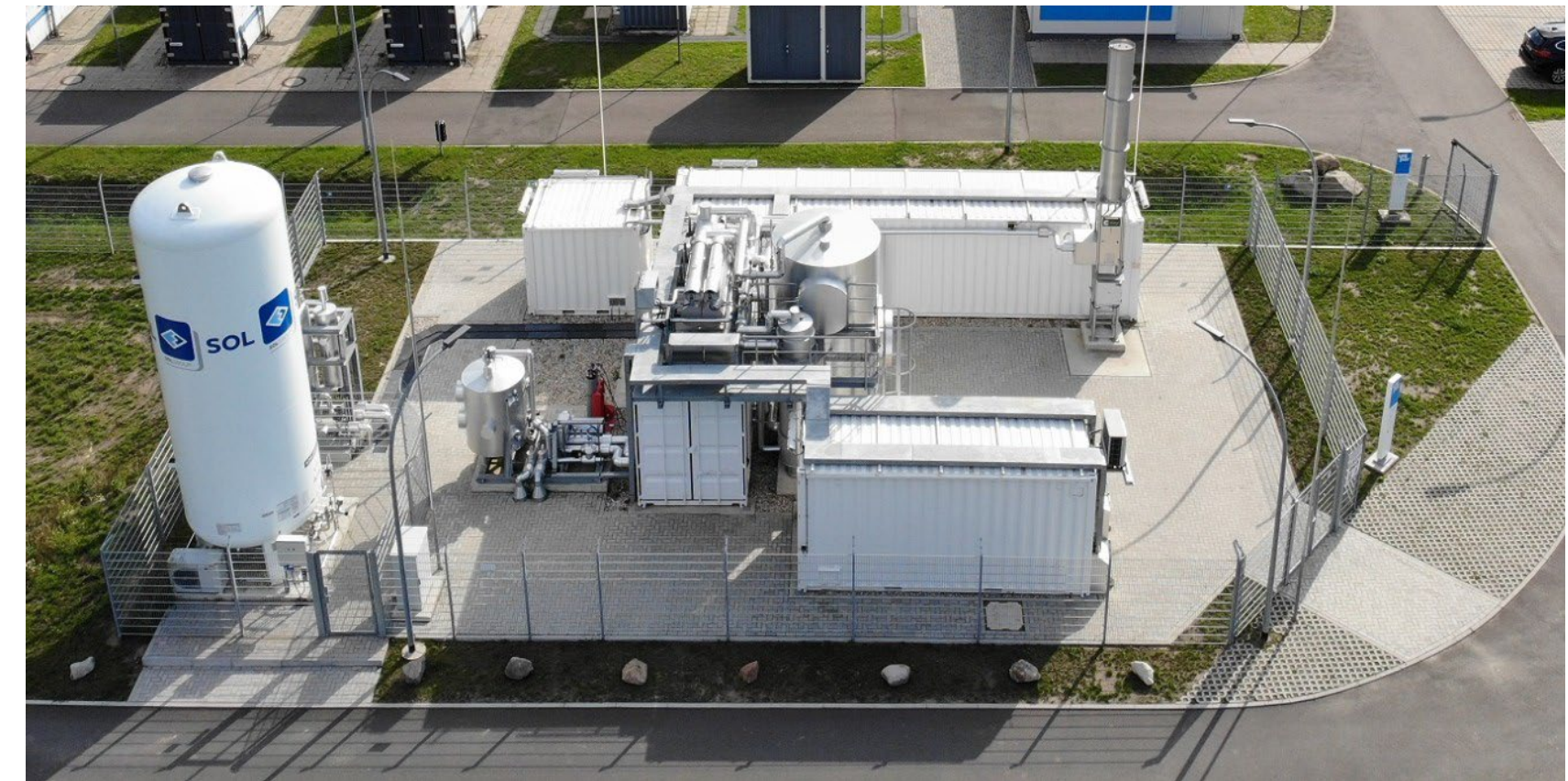
CO 2 methanation plant (Falkenhagen, Germany)
